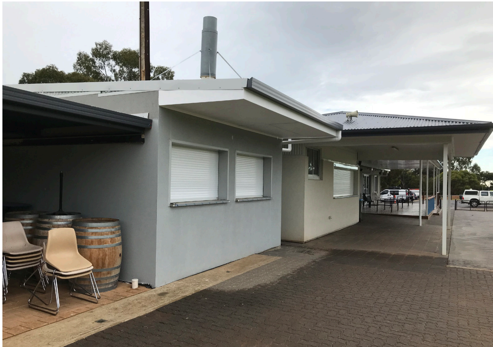
Photo: New Outdoor Kitchen and Gymnasium Block at St Marys Sports Association Oval
